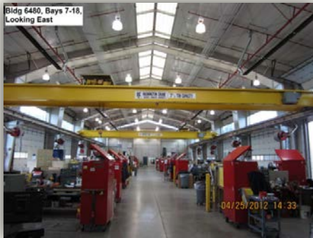
Camp Withycombe Industrial Lighting
