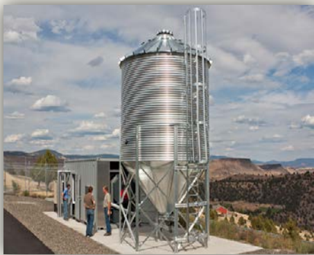
Biomass Pellet Boiler
