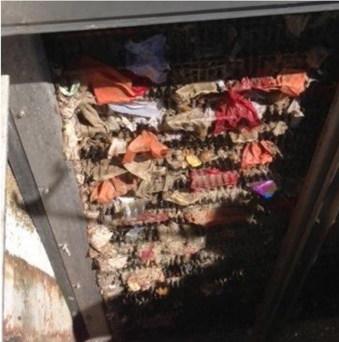
Figure 2 – Westside Wastewater Treatment Plant screens May 3, 2015
